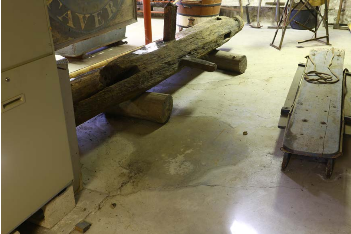
Fig. 26. The dark stain on the floor is evidence of past/recent water. The source and cause of this is not known. The cellar should be periodically monitored after snow melt and heavy rain to understand how it reacts when subject to large amounts of water. No water was observed at the time of the building survey.
