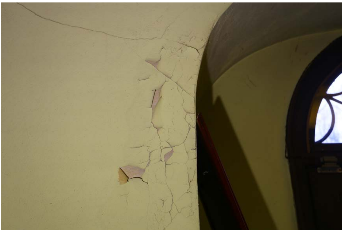
Fig. 29. Localized area of failing paint at the north entry.
