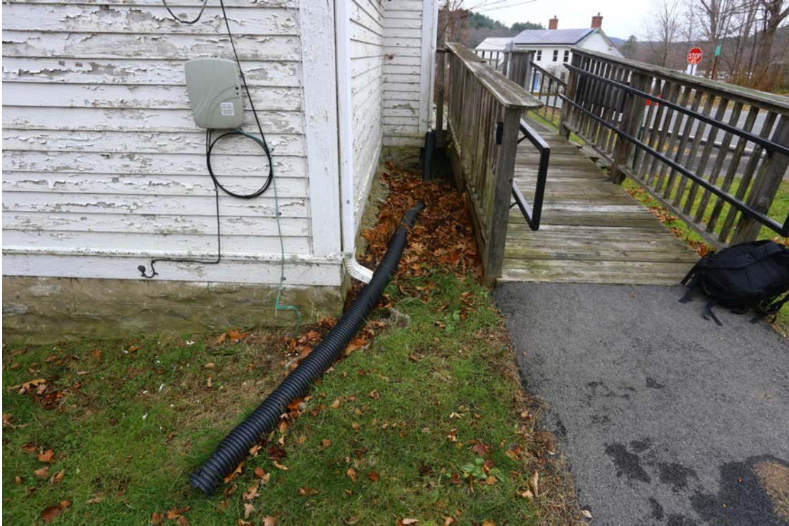
Fig. 21. Northeast corner of the building looking west. Flexible piping carries runoff from the leaders flanking the entry, preventing discharge immediately against the building. Connecting the leaders to a subsurface pipe run to daylight would improve the appearance of the building and provide a more durable, long-term solution for controlling runoff.
