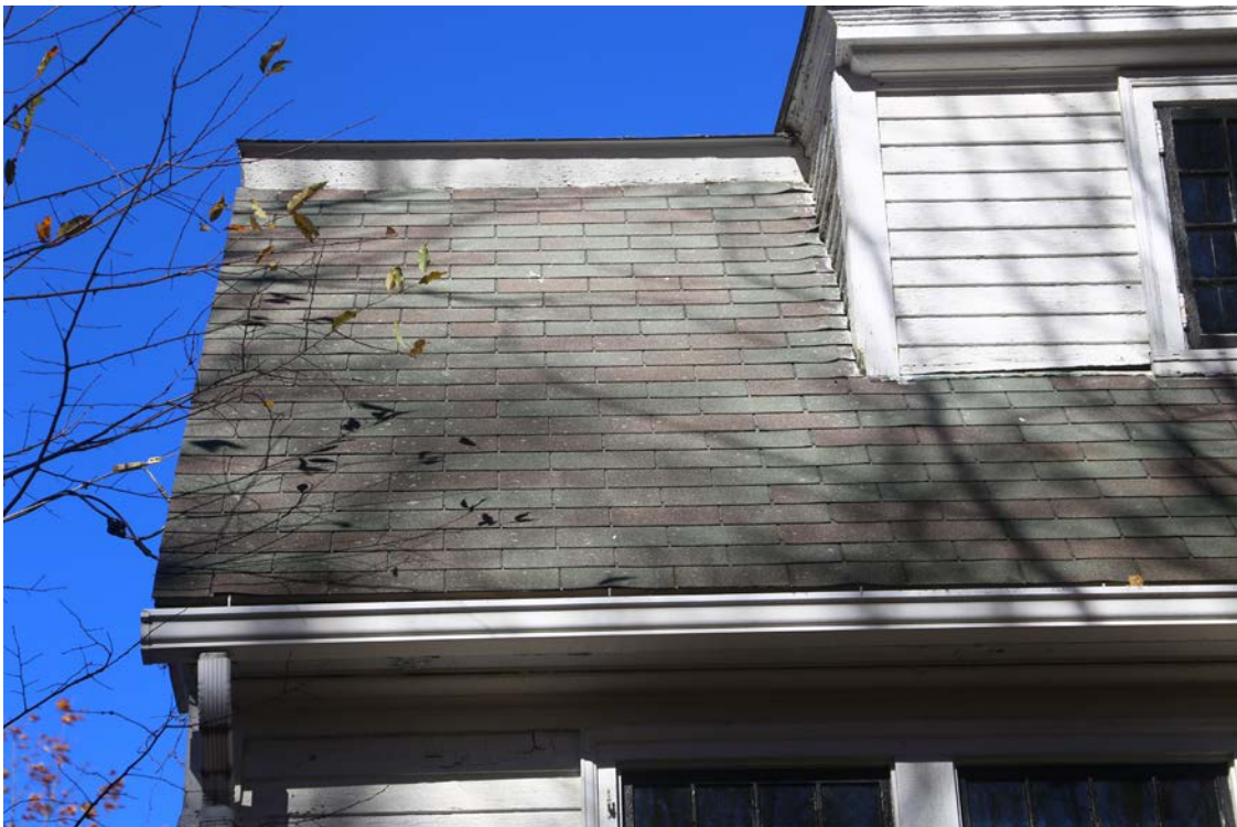
Fig. 7. South elevation, west end. Shingles on the south side of the building, which receive direct sunlight, do not have lichen growth or surface staining. Although the surface condition is better than on the north side, the shingles are nearing the end of their service life and should be replaced soon.
