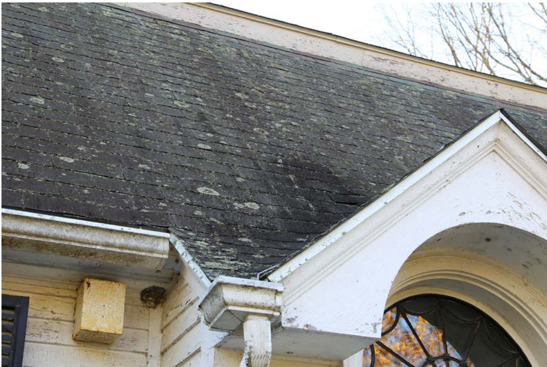
Fig. 5. Detail of the north roof, lower pitch showing lichen and staining on shingles. Note the condition of the gutters and woodwork.
