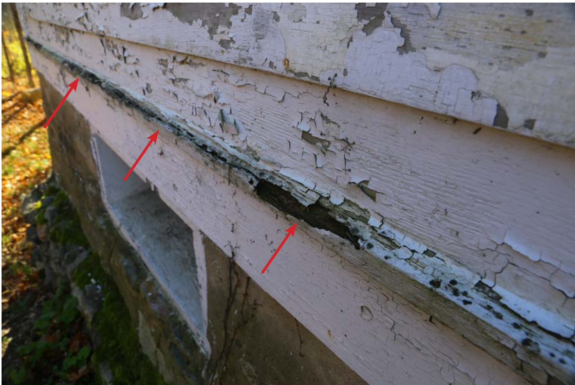
Fig. 12. East elevation showing rotted area of drip mold. The drip mold should be removed and replaced with new material.
