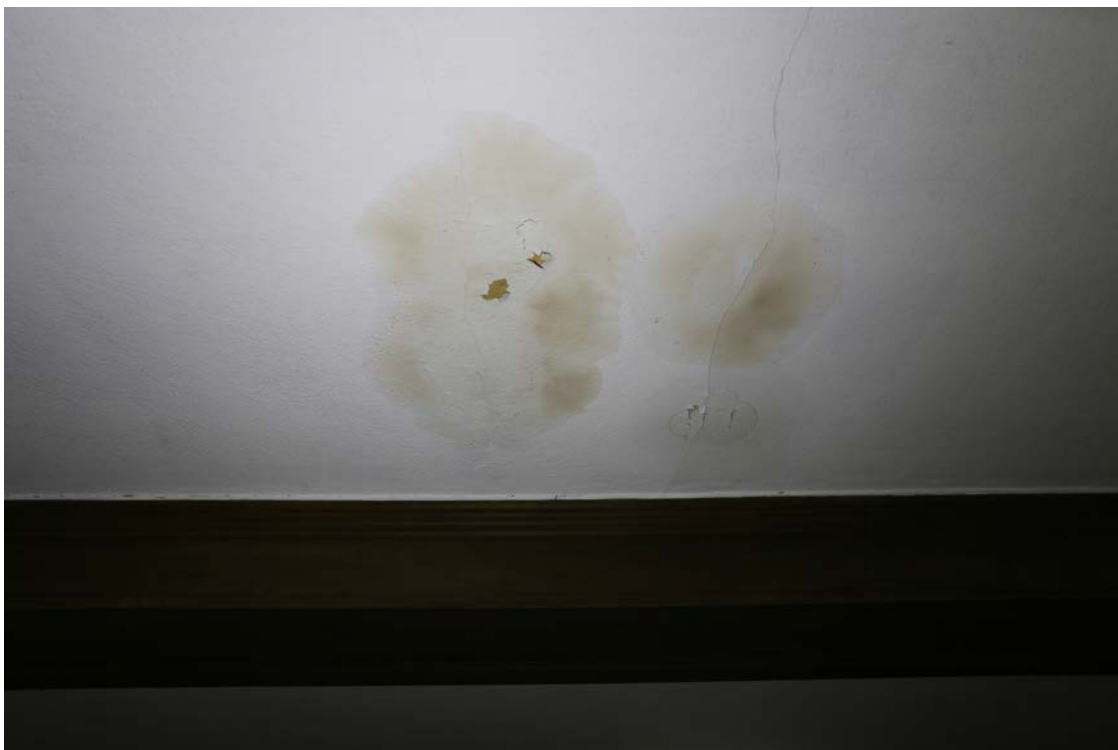
Fig. 33. Cracks, patches and stains on the first floor ceiling.
