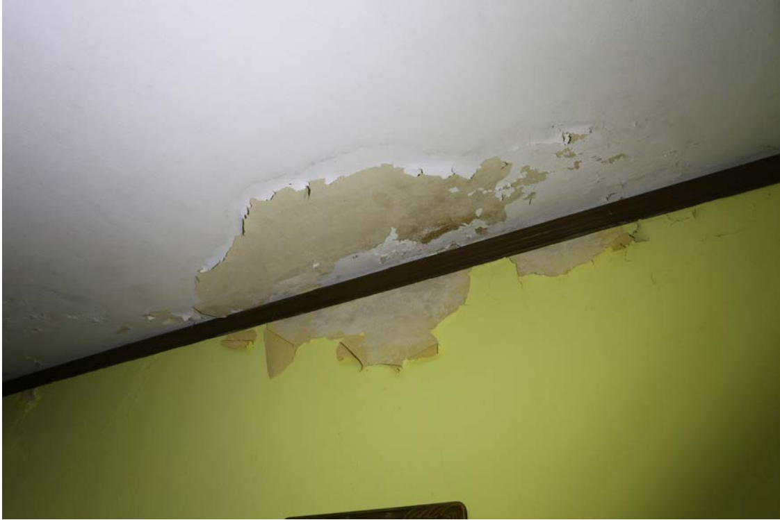
Fig. 30. Water damaged paint and plaster above the fireplace. This appears to be old damage and not from active leaks.
