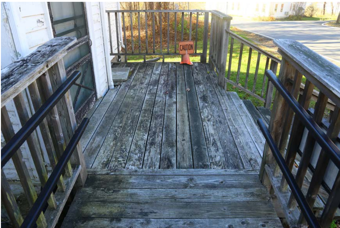
Fig. 22. Committee members have commented that the wood decking is extremely slippery when it becomes wet. Various parts of the decking and posts are rotted and in danger of failing if weight is put on them.
