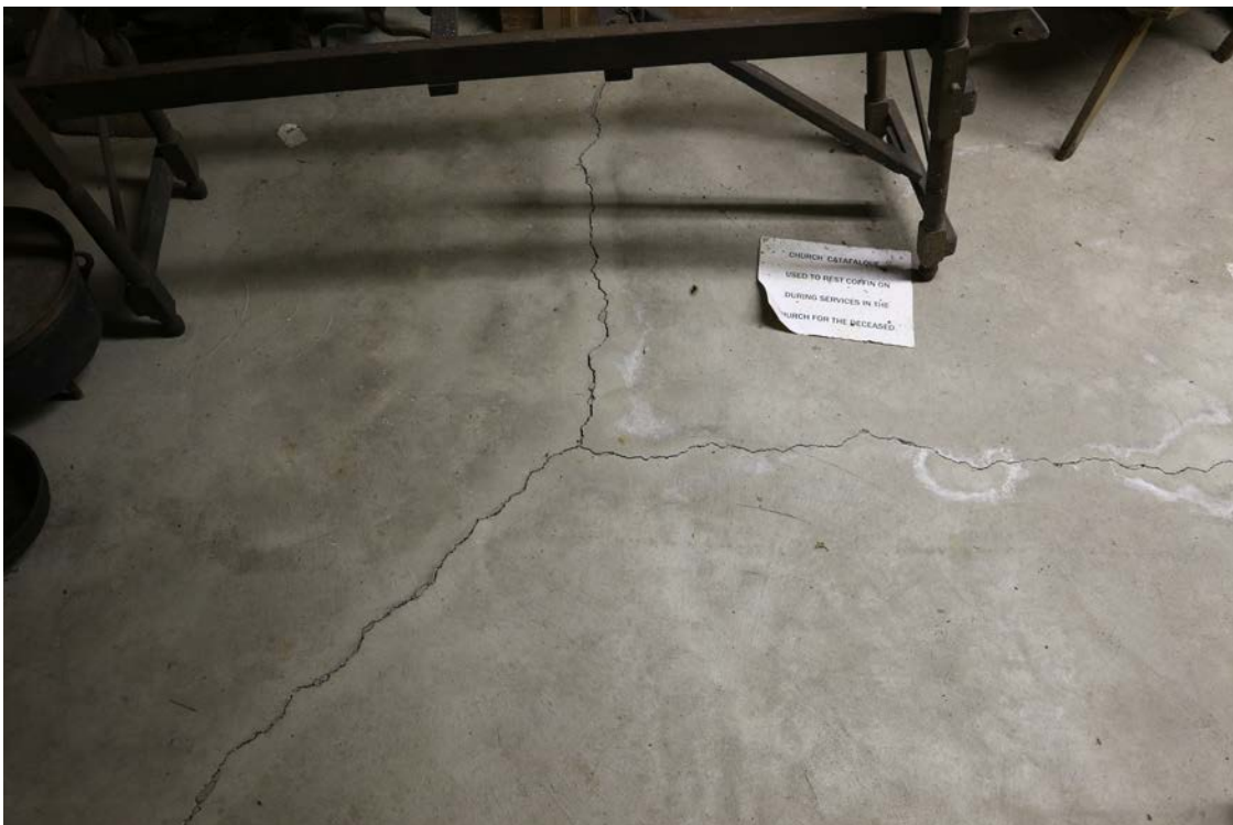
Fig. 27. Random cracks are present in the floor slab. Aside from allowing ground water into the building (note stains), they are not a matter of great concern.
