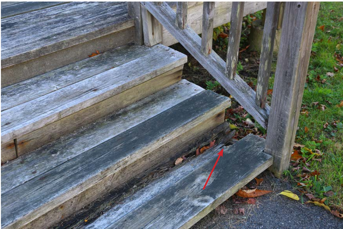
Fig. 24. Detail showing rotted stair tread. Many of the posts are deteriorated where they meet the ground and are in danger of failing if weight is put on them.
