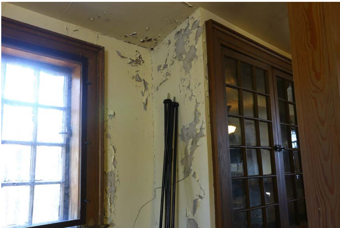
Fig. 32. Second floor, south elevation. Failing paint and plaster appear to be the result of water infiltration associated with past roofing and/or flashing failures in this area. These issues do not appear to be active.
