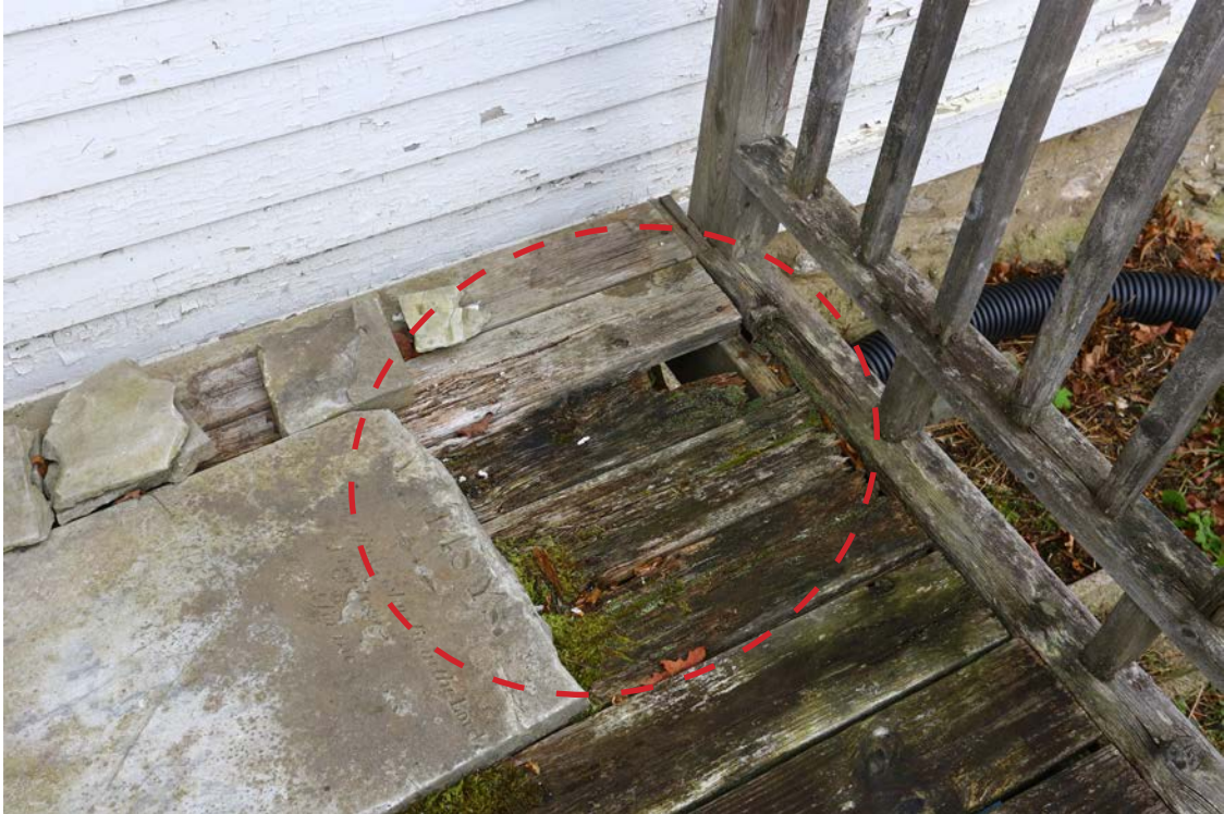
Fig. 23. West end of the deck showing area of severely rotted boards.
