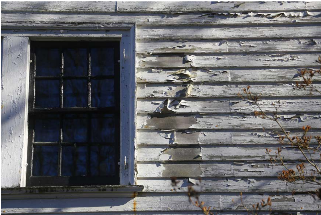
Fig. 14. Another example showing paint failing to bare wood. A thorough scraping of the building, followed by the application of a high-quality primer, will prepare the siding for repainting.
