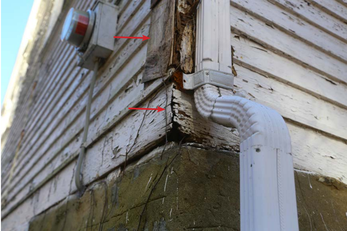
Fig. 11. Southwest corner. The lower portion of the corner of the building here is rotted. The siding and watertable needs to be removed to determined the full extent of repairs. The deterioration appears to be localized to the lower 3'-4' of the corner.
