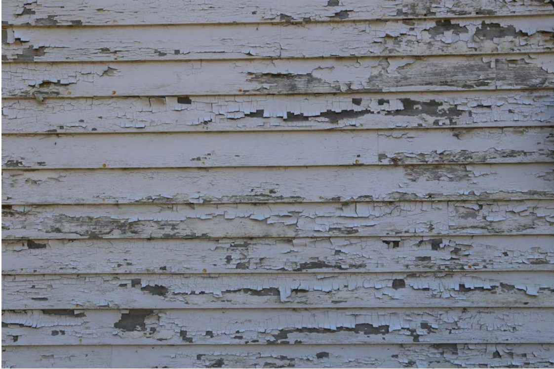
Fig. 13. Representative example showing the typical condition of the exterior paint finish. The majority of the clapboards and wood trim remains in good condition, with only the paint finish failing.
