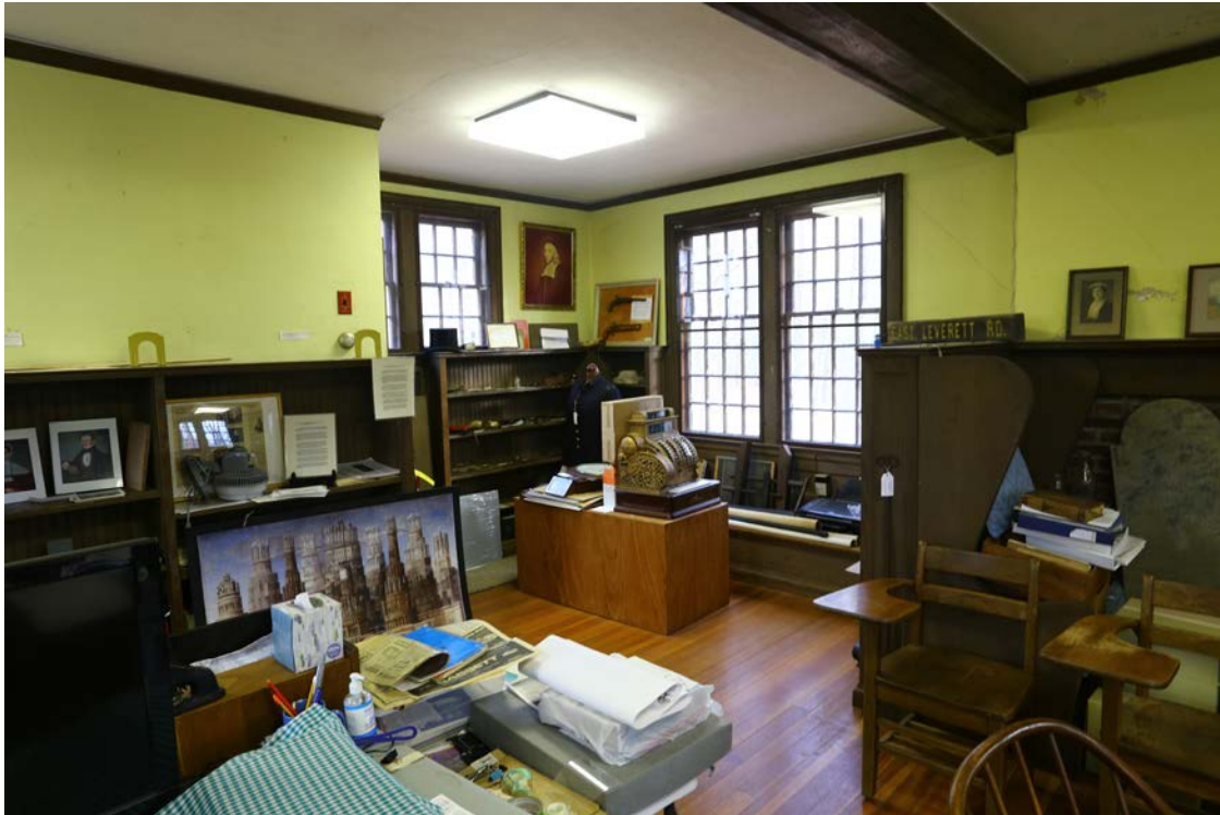
Fig. 36. Example of the first floor ceiling fixtures. The light fixtures are dated and should be replaced. Improved lighting should be installed throughout the building. Consideration should be given to fixtures that are both functional and appropriate to the building's aesthetic.
