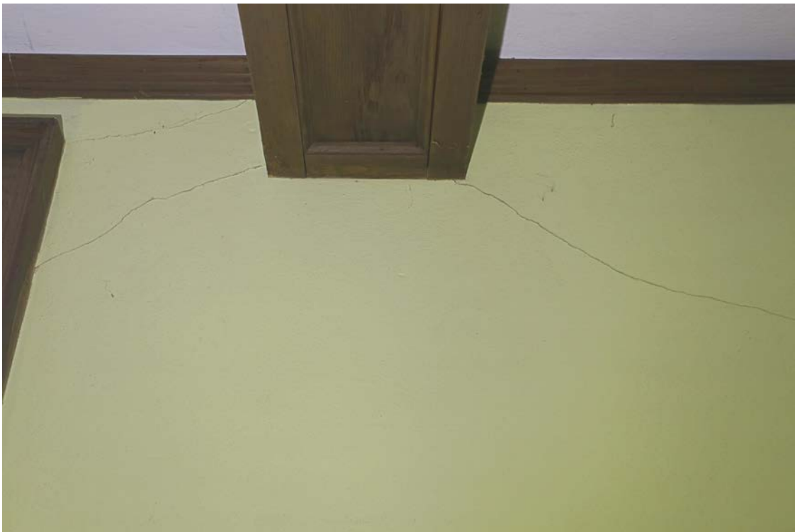
Fig. 31. Cracks radiating from the north end of the west ceiling timber on the first floor. No obvious movement/displacement is present and the surrounding materials appear to be in good condition.
