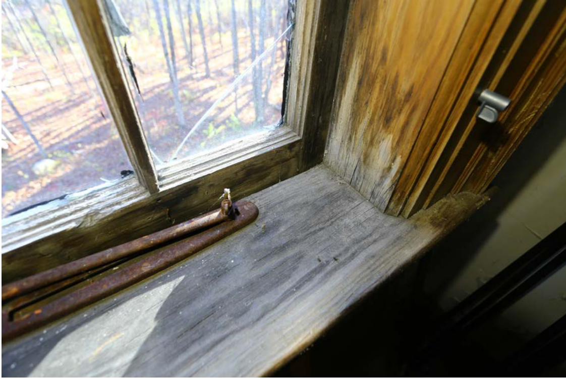
Fig. 34. The woodwork trimming and finishing many of the window openings suffers from UV damage and, in some cases water damage. The woodwork should be prepped and finished with a high quality clear coat or paint finish.
