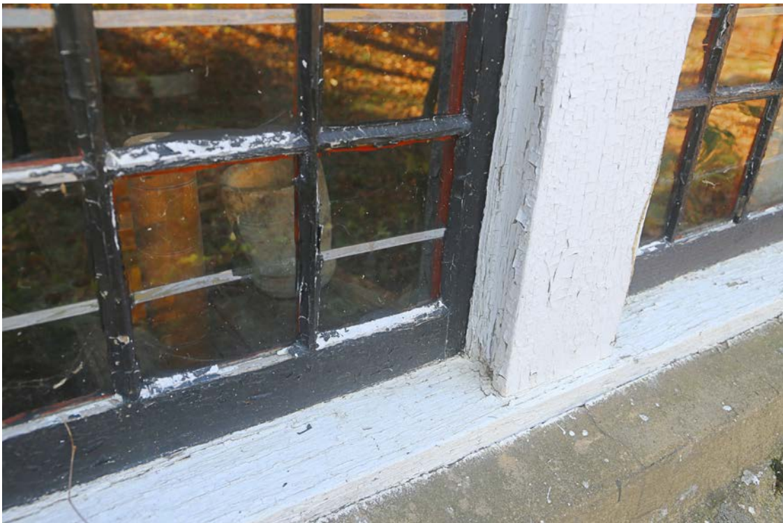
Fig. 16. South elevation, west cellar windows. Detail showing deteriorated glazing putty and failing paint. The interior surface of these sash have been damaged by rodents.
