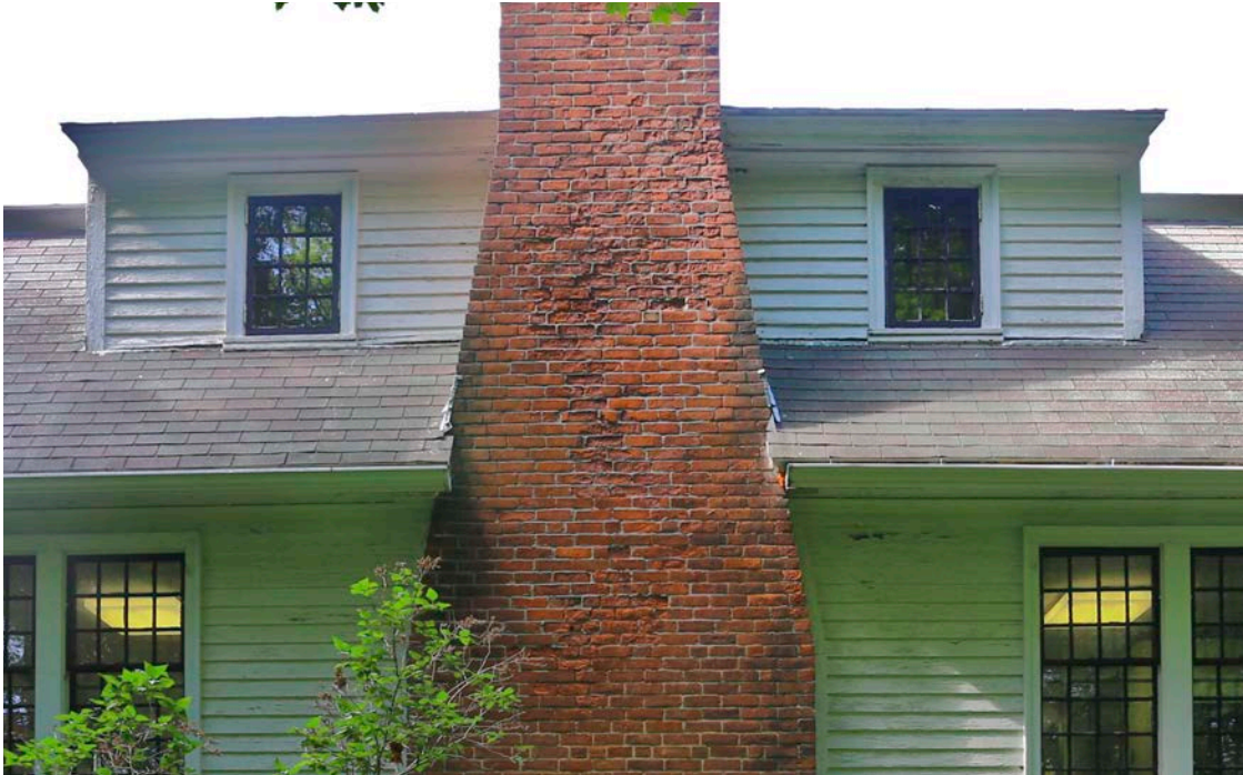
Fig. 8. South elevation. Detail of the chimney identifying an area of deteriorated brick. While unsightly, the brick appears to remain structurally sound. Closer inspection, including probing of the exposed brick surfaces, is recommended to confirm condition. As the fireplace is no longer active, the chimney currently serves only to vent the furnace. The flue should be inspected to determine its condition and suitability for continued use.
