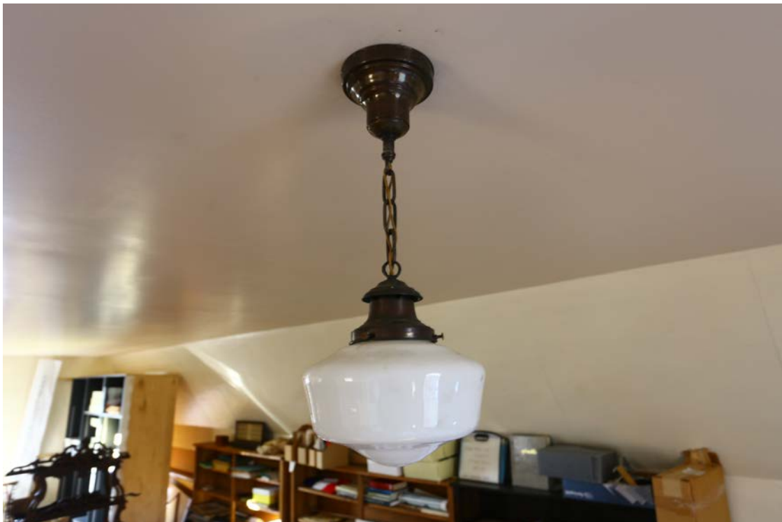
Fig. 37. Second floor ceiling fixture. These fixtures are likely original to the building and remain in service. They are served by cloth-covered wiring, suggesting the wiring may date to the construction of the building. The fixtures are fine examples of their period and should be rewired if they are to remain in use.
