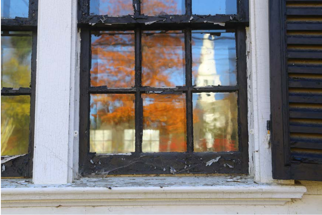
Fig. 15. Typical condition of the window sash paint and putty. The wood frames remain sound.
