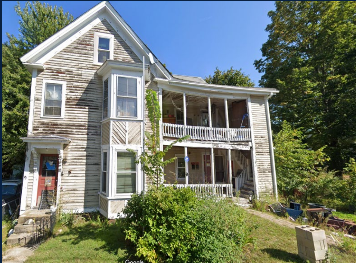
Property in Violation of State Sanitary Code
